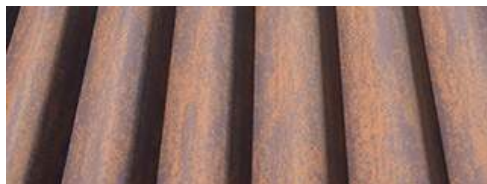
PAINTED RUSTED ROOFING
