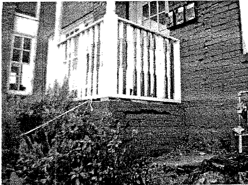
Brick work to be repaired.
