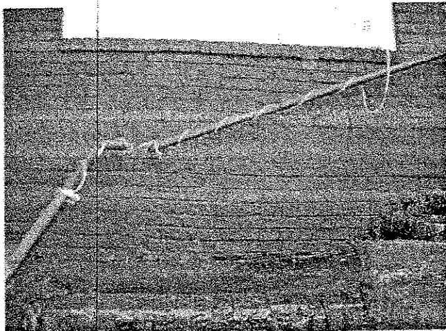
Settlement of the brick wall
