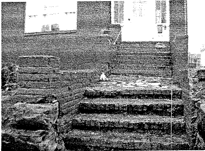
Brick work to be repaired.
